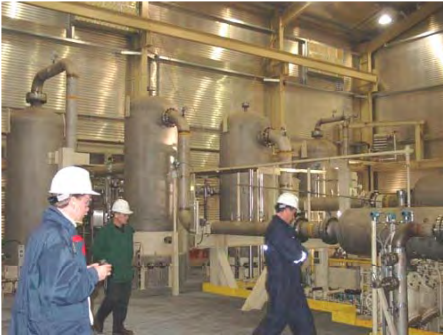
The CO 2 - compressor facility
